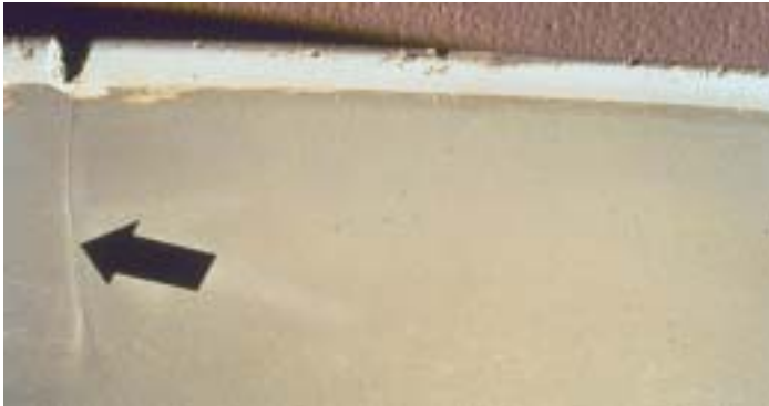
A prop in the process of failing. Note crack.
