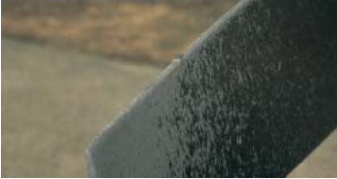
Blade erosion: Bare metal corrodes rapidly. Keeping blades properly painted is inexpensive routine maintenance.
